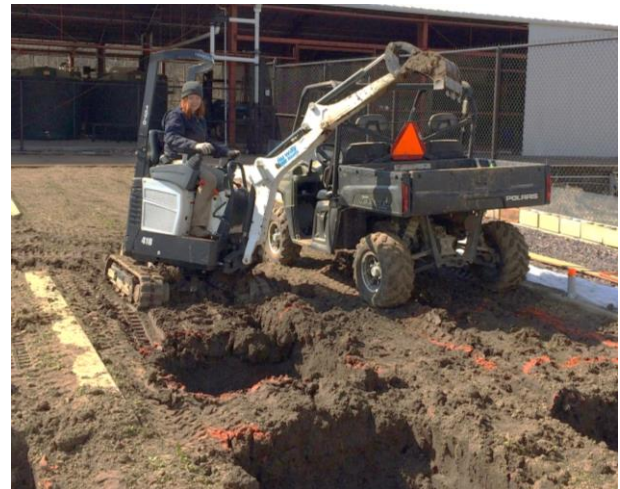
Digging perfectly spaced squares for experimental communities of prairie plants under differing soil microbe conditions
