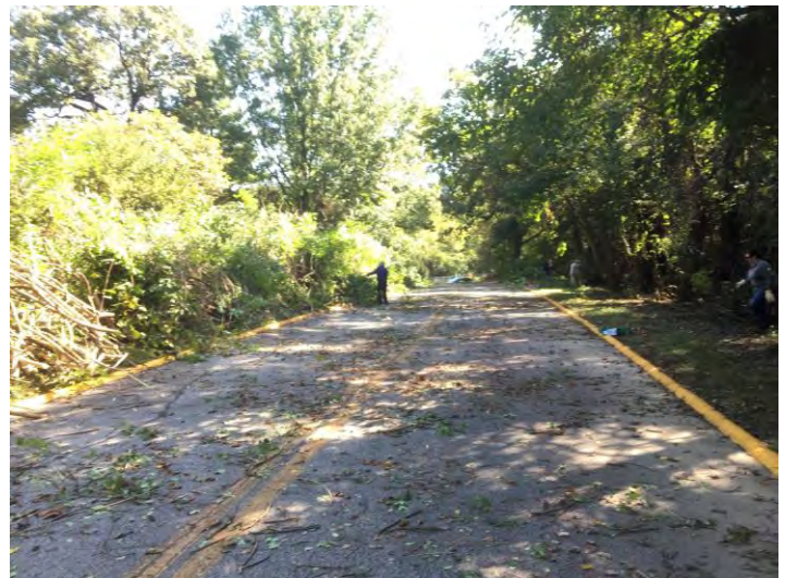
A 500-foot long , half-acre area of invasive bush honeysuckle was cut, moved, and stacked for disposal on the lawn across the road in a few short hours.
